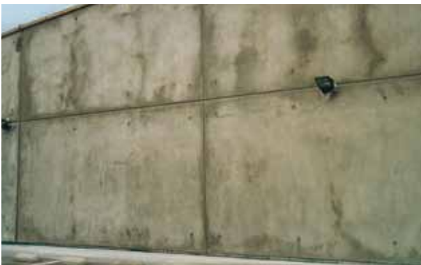
New concrete with severe blemishes
